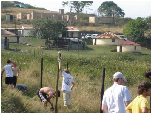
Students from Malvern Prep work on building a fence in a project with the Hillcrest AIDS Center
